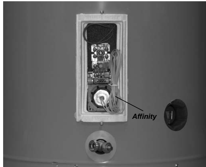
Thermistor Wires Connected to TB (3 and 4) on Affinity Control Board
